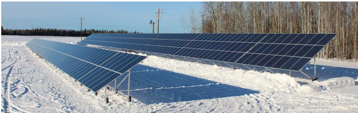
Figure 6: Solar PV array installed in Fort Simpson which is 130 km northwest of Fort Providence. Photo from the SkyFireEnergy website.
