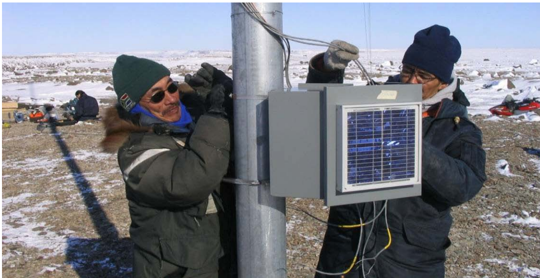
Figure 1: Alan Pogatok and William Hurst are shown installing the wind monitoring station on the East Ridge. Joseph Kuptana is in the background.
